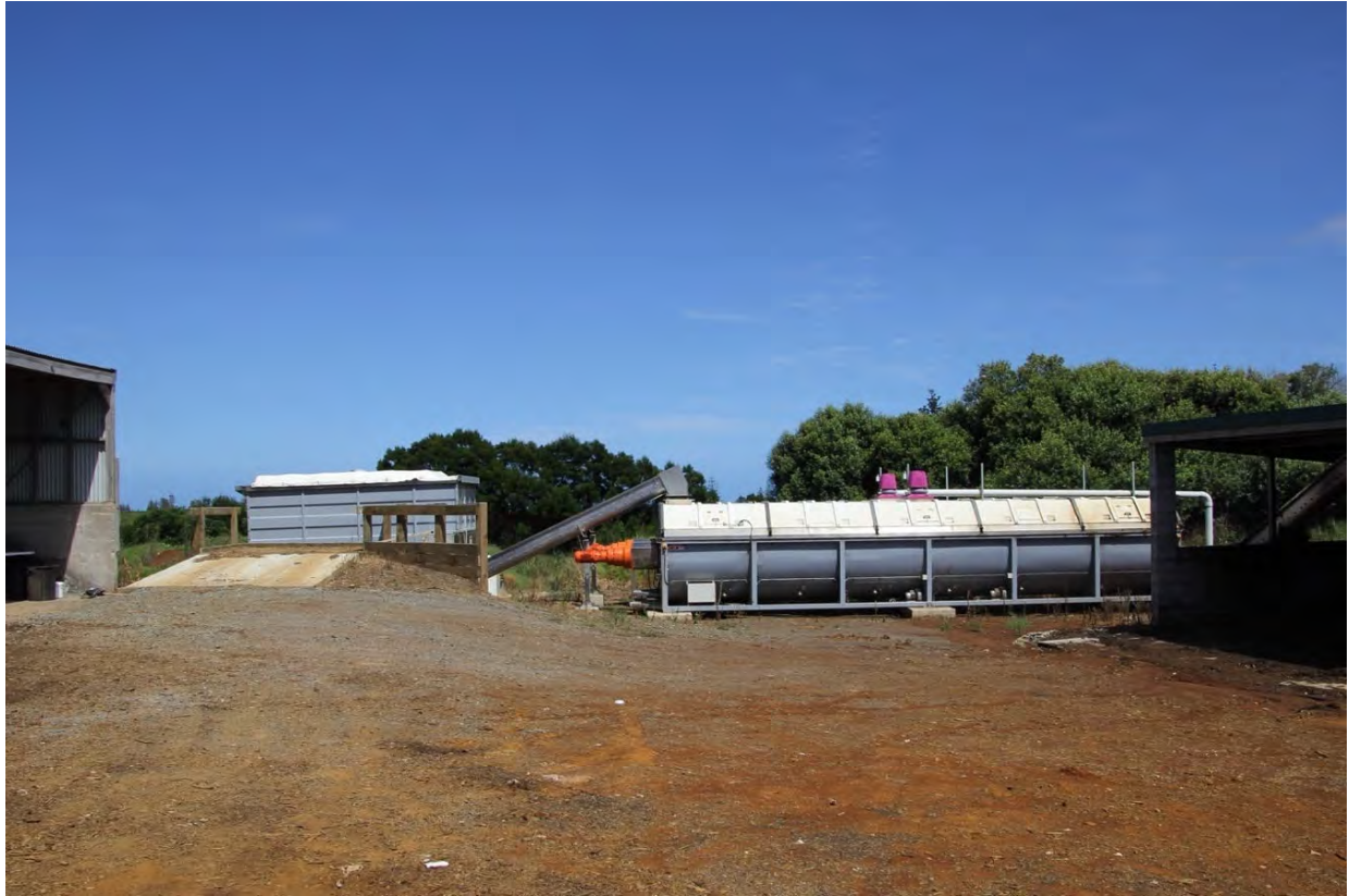
Figure 3.13: HotRot Compost System behind the WMC facility
